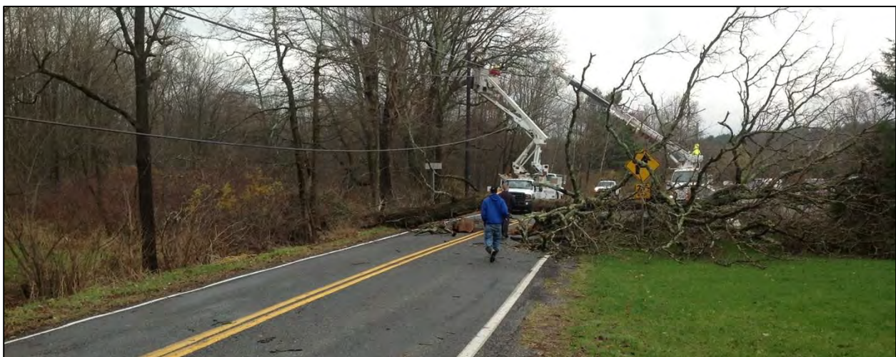
Figure 27 - Fallen Trees are Cleared from Powerlines Following Superstorm Sandy
