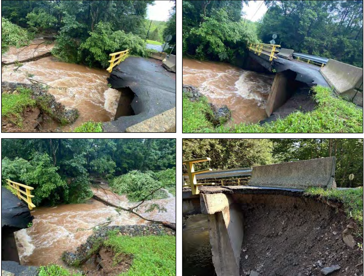
Figure 24 - Paradise Township Bridge Collapse
