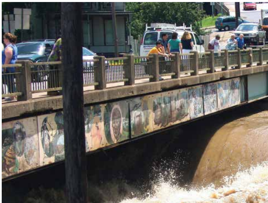
Flood event conditions of the McMichaels Creek in Stroudsburg
