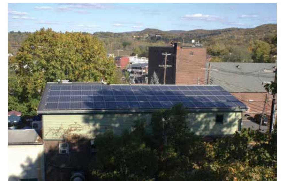
Solar panels over the Sarah Street Bar & Grill
